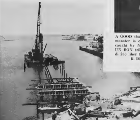
LAGO'S NO. 3 Finger Pier, above, begins to take shape as the first concrete caps on pilings are fitted. The area near the police station in Oranjestad, below, takes on a new look with new traffic islands. FINGER PIER No. 3 di Lago, ariba, ta cuminsa haya forma cu sintamento di e promer cabazonnan di concreto bashá ariba e pilanan. E vecindario banda di warda di polis na Oranjestad, abao, ta haya un aspecto nobo cu e islanan nobo di trafico.
